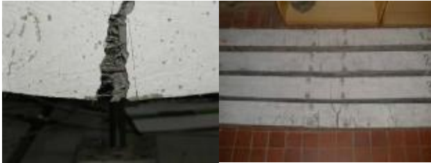
Figure. 14 a) Detail of the failure mode of the tested beam with fibres and steel bar reinforcement and b) crack patterns of the tested FRC beams
