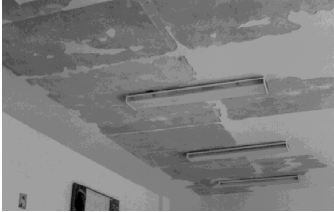
Fig. 7.3 Damaged plasters in the classroom.
