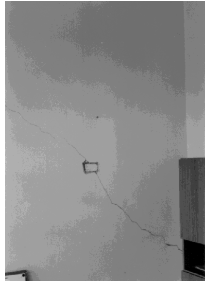
Fig. 7.4 Cracks in partition walls
