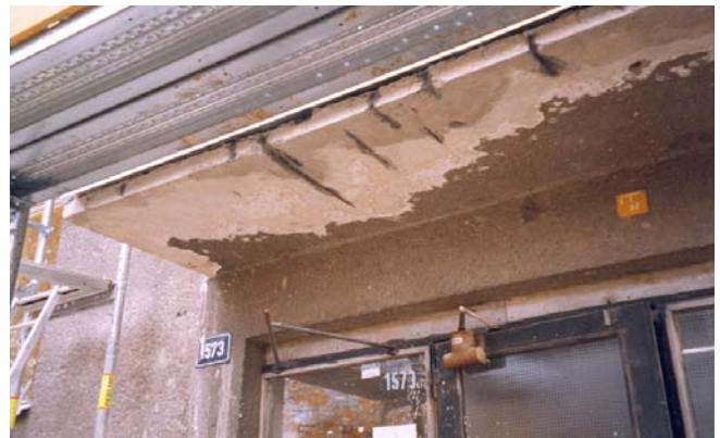
Fig. 7.6 Deterioration of balcony.
