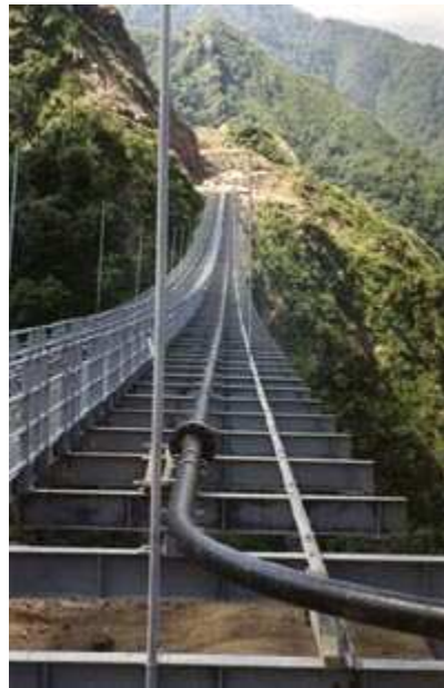
Figure 5. Slurry pipeline through rugged isolated area in Andes, South America (source: website Pipeline Systems Inc.).
