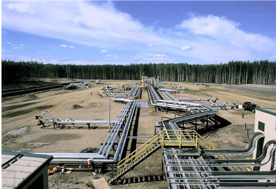
Figure 4. Processing plant with supplying pipelines handling tar sands and crude oil in Alberta, Canada (source: website Syncrude).
