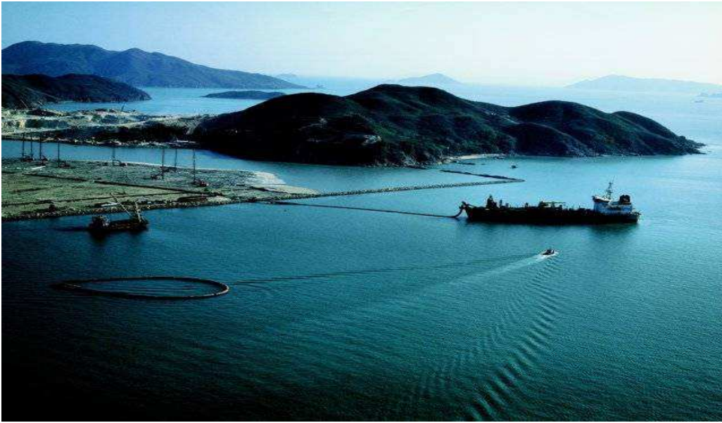
Figure 3. Trailing suction hopper dredger supplying a shore slurry pipeline.
