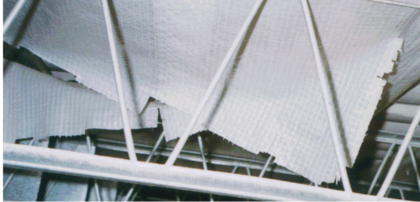
Fig. 2 Leakages in the wind barrier
